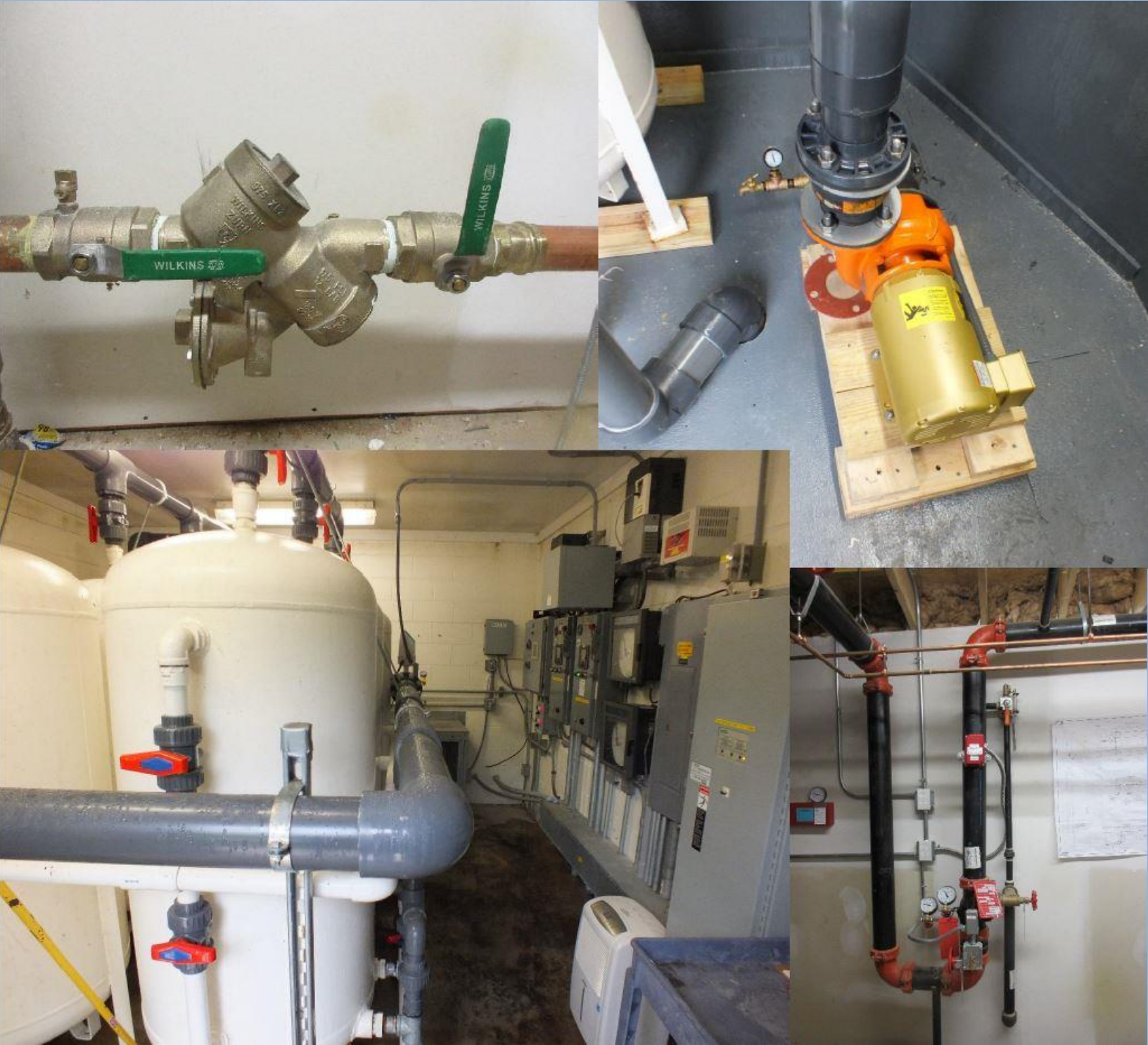
Pictured above: small public drinking water system infrastructure
